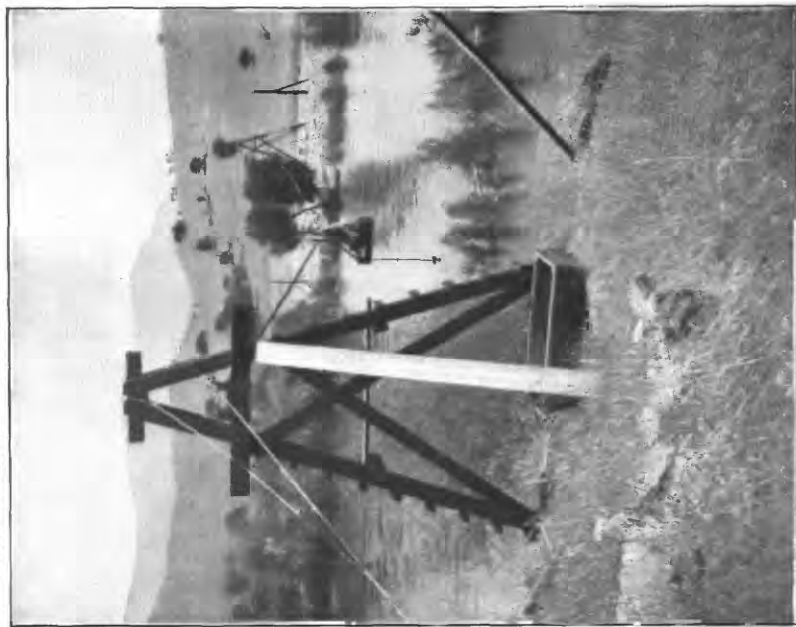
A. CABLE STATION, KINGS RIVER, NEAR RED MOUNTAIN, CALIFORNIA.
